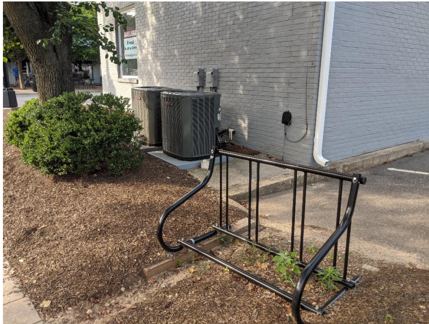
AC Units and Bike Rack Located on the West Side of the Building
